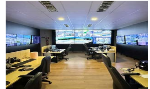
Fire Monitoring Center
